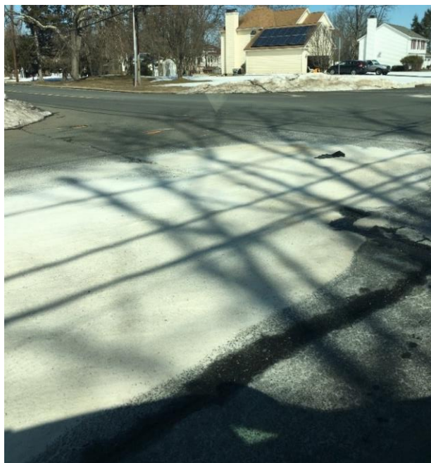
Figure 6: Excess road salt piles up at an intersection in Ewing, NJ (Feb. 26, 2021). Some salt-spreading trucks continue to unload salt while stopped at an intersection or around turns, leading to large piles like this one that remain on the road until the next runoff event. One road salt BMP that is easily implemented and saves money for the salt applicator is to turn off spreaders while the truck is idling.
